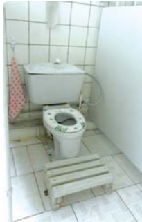
Broken flush tab
